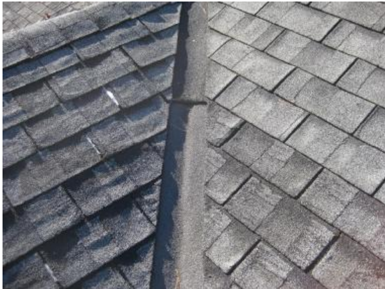
Shingles are cracked and curled; indicating they are older. Recent repairs to the valley are evident.
